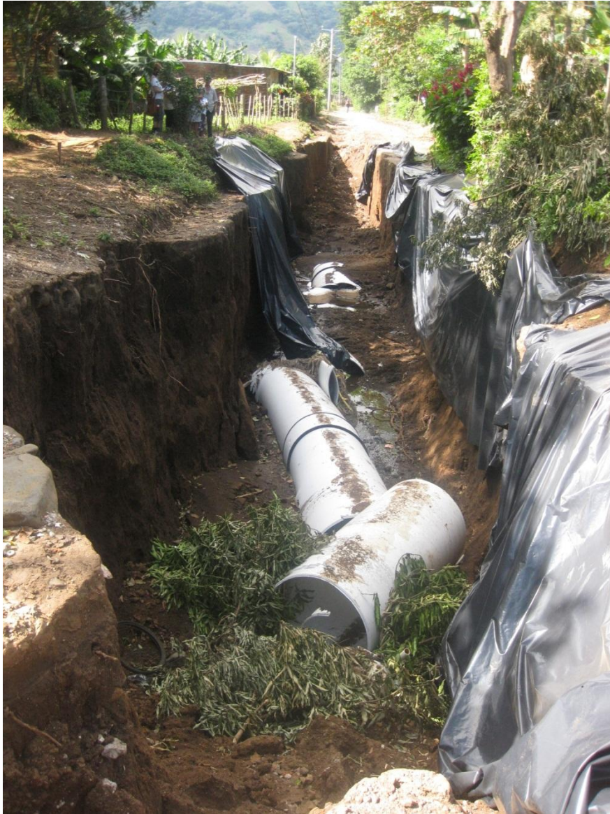
Figure 7: Water pipes damaged by the floods along the Calle central alsause road (along the border of Malaga and Traveras), 26 th October 2011
