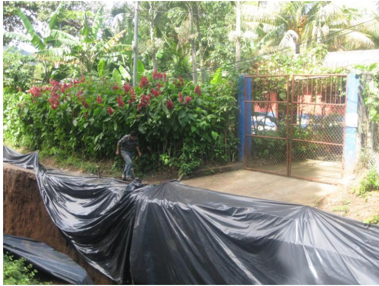
Figure 8: The road outside this house has collapsed.
